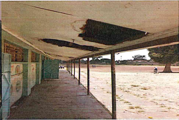
Figure 2: worn out ceiling boards at Juja road ECDEs
