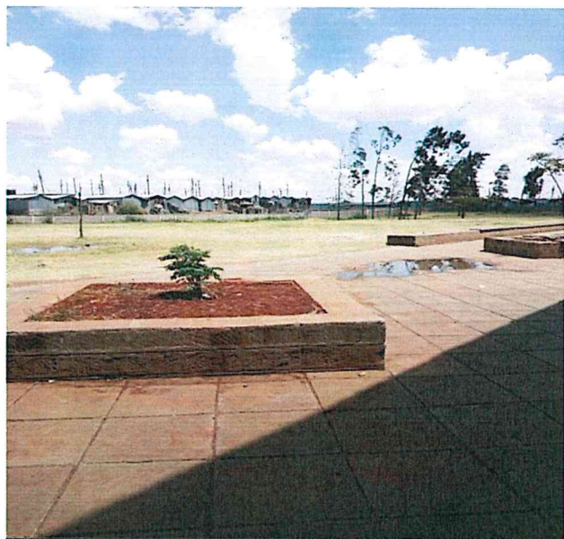
Figure 2: Incomplete Perimeter wall at St. Elizabeth Primary
