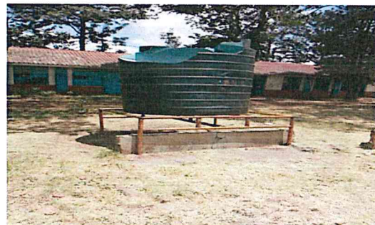
Figure 2: Broken Water Tank at Muslim Primary
