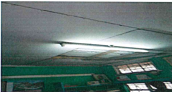
Figure 1: worn out ceiling board of the office of Muslim Primary
